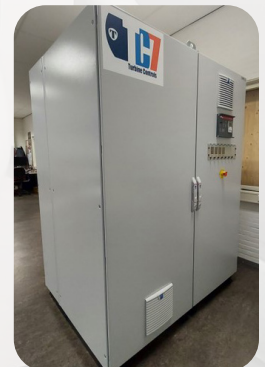
TC7 CONTROL SYSTEM
